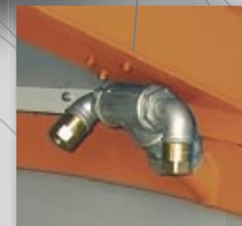
Water distribution ring with high efficiency spray nozzles.
