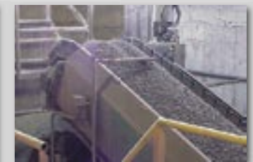
Apron conveyor transporting hot materials from kiln/cooler system.
